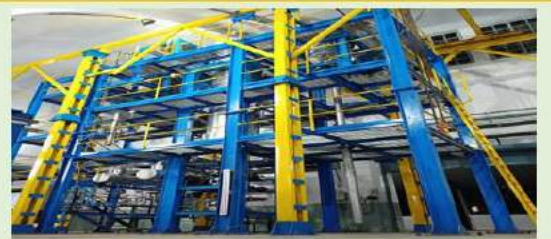
Fluidized Bed Gasification Pilot Plant
