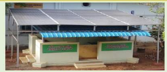
Solar Powered Hydrogen Generator (500 L/h)
