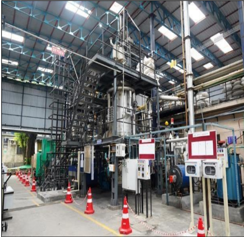
The 5 kgph hydrogen oxy-steam gasification system
