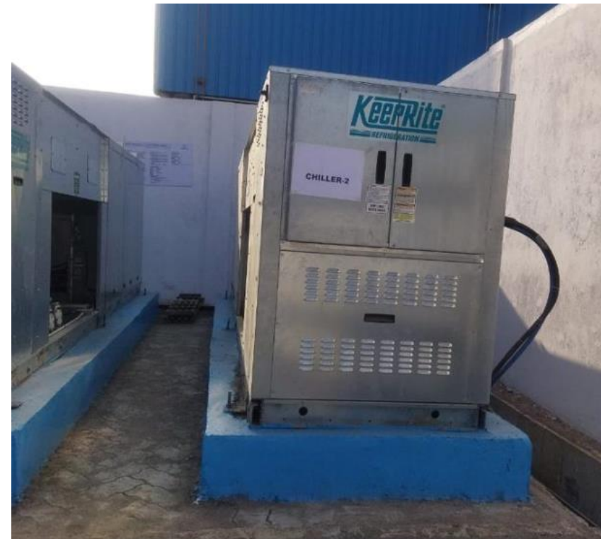
Dispenser- Chillers installed at Site
