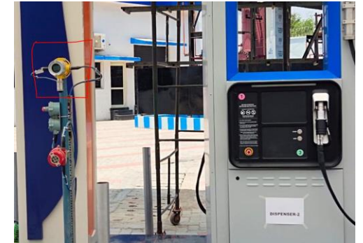
Gas Detector – Dispenser 2
