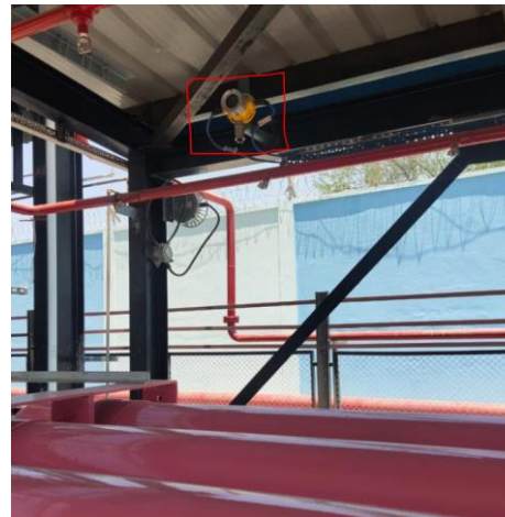
Gas Detector – HP Storage Tubes
