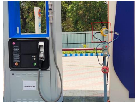
Gas Detector – Dispenser 1
