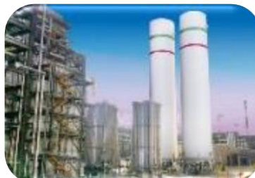
ENGINEERED TANKS ~ 1000M 3
