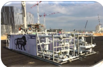
MULTI-CORE H 2 / HE VJ TRANSFER LINES (ITER)
