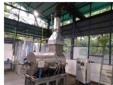
H 2 S incinerator
